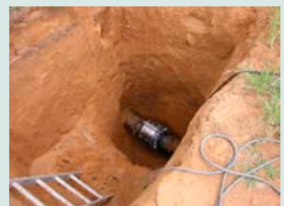
Teletest tool on pipe in bell hole
