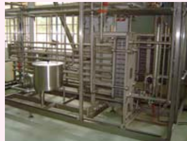
Plate type heat exchanger sterilising system
