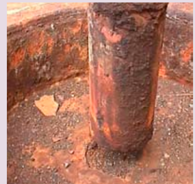
Corrosion damage in tank floor
